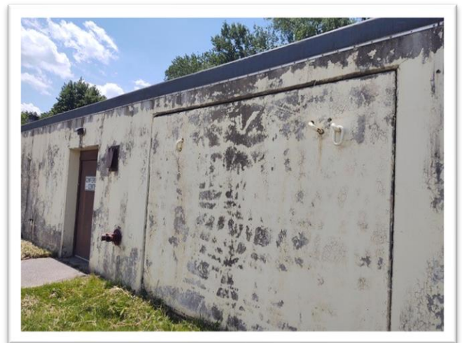
Outdoor bomb blast shelter
